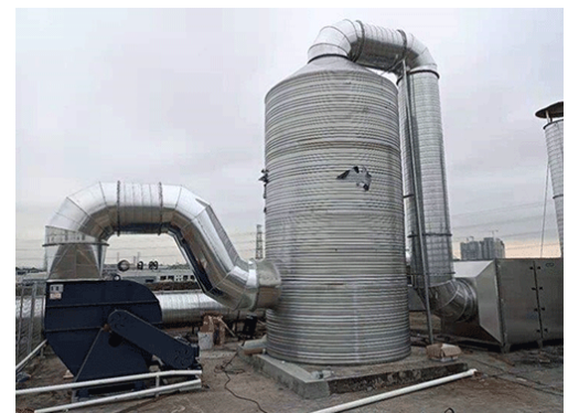
Brother Technology (Shenzhen) Ltd.: VOC treatment system
